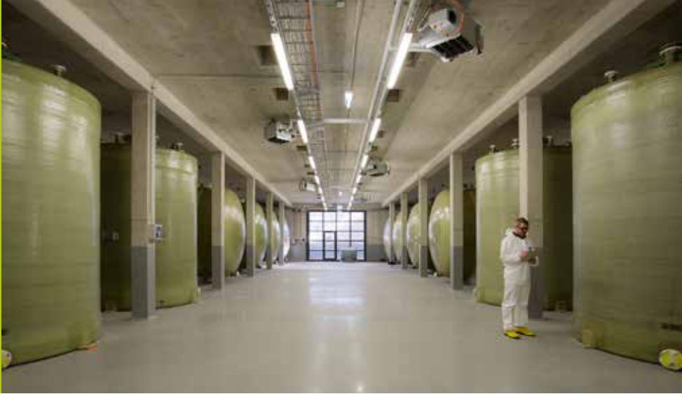
Redox flow battery.
